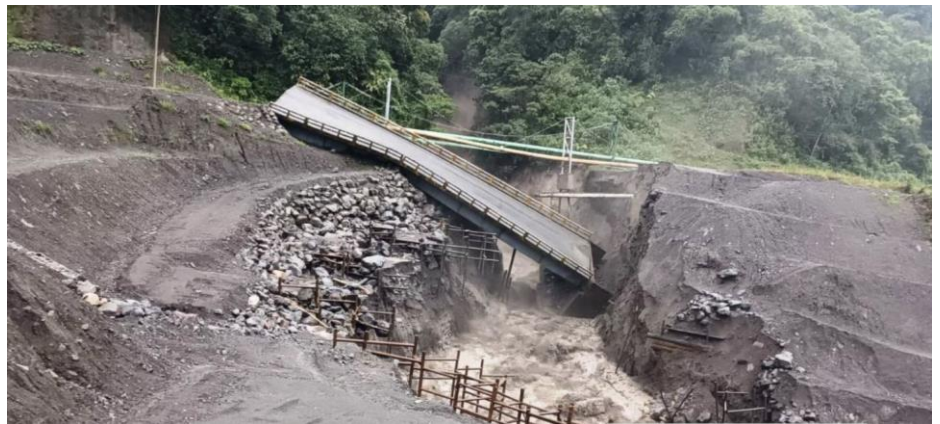
This bridge out in the eastern jungle collapsed in February.
