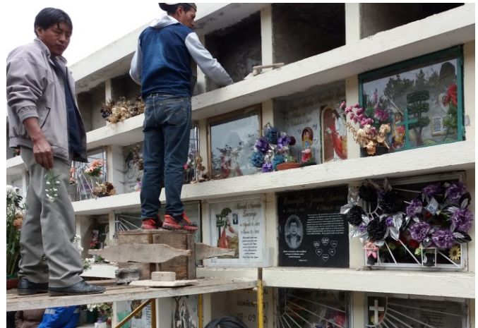
Workers cementing in the niche during the funeral, after placing the casket
